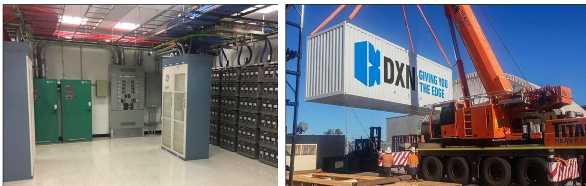
Figure 5: Cable Station Equipment & Modular Cable Landing Station
